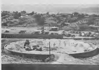
A SOLID packed base of sand is needed for a round tank's foundation. The two-tone tanks at right both reflect and absorb the sun's heat.
